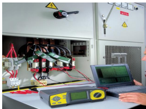
Figure 3. Multiple equipment's METREL used for active power measurements
