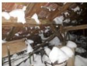
Fig.1 The state of the roof of the
