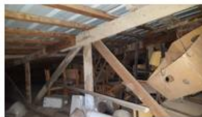
Fig.2 The state of the roof of the Ernest Koliqi school, Ferizaj Esat Mekuli school, Podujevë
